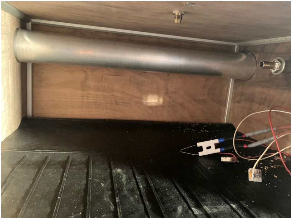
Figure 2: Interior view with ignition electrodes
